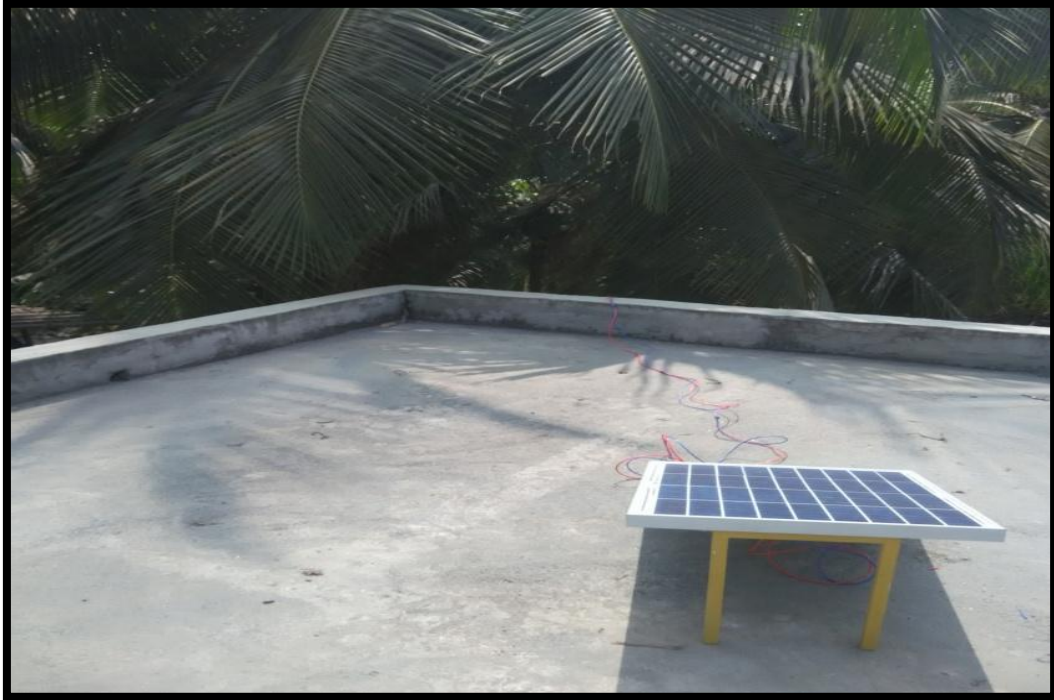
Solar panel installed in project site
