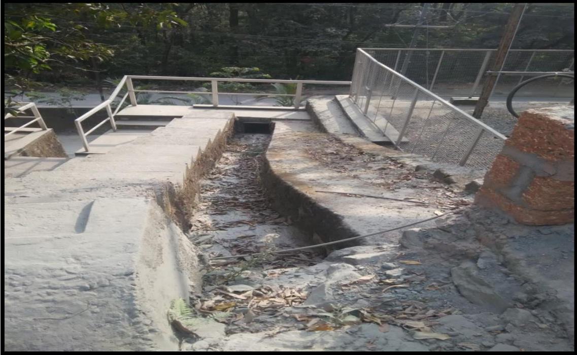
Garland drains for storm water management
